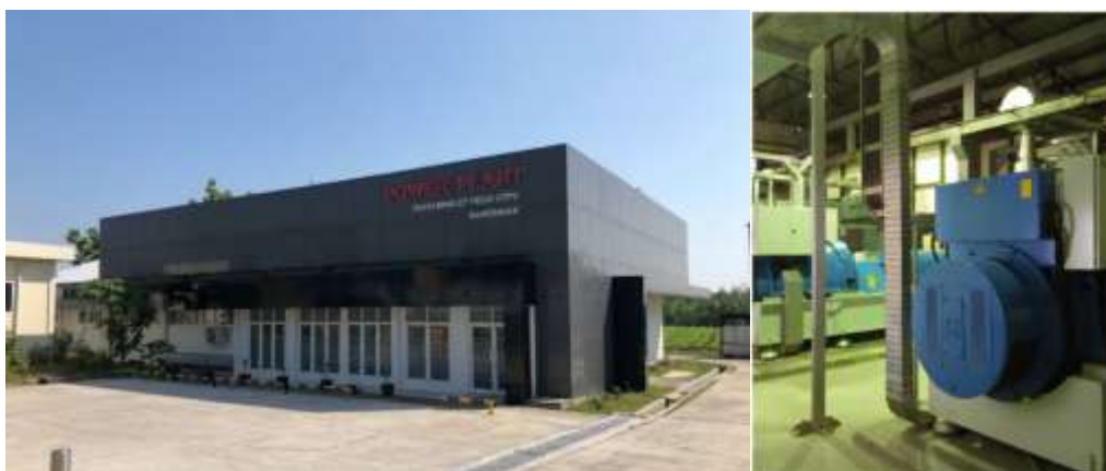
Figure 3. DRUPS facilities at the Kawengan Power Plant, Cepu Area
