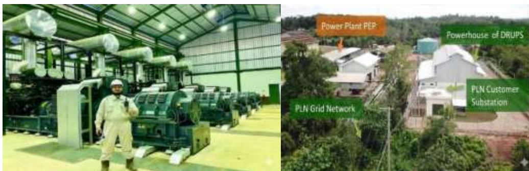
Figure 4. DRUPS facilities at Tanjung Power Plant, South Kalimantan
