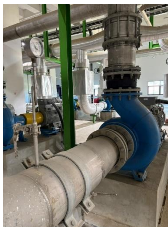
Figure 5. Pressure Gauge Position
