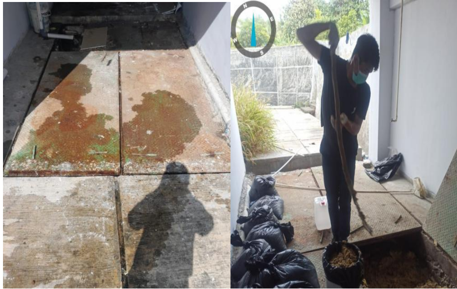
Figure 4. Grease trap Pictures & Grease trap Maintenance Process Pictures at RS X
